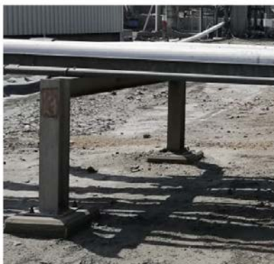
Pipe sits on station not clamped
